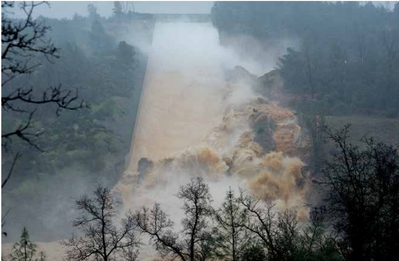
The Oroville Incident, Feb. 2017. As the Oroville Reservoir main spillway crumbles, mud, rocks and concrete flow in to the Feather River on February 8, 2017. Source: Bill Husa, Chico Enterprise-Record.
