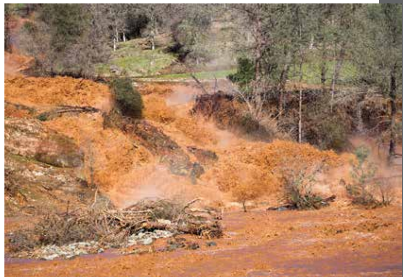
Oroville Dam Spillway Erosion, Feb. 11, 2017. Water and debris from the emergency spillway failure flow into the diversion pool just downstream of the dam. Source: Dale Kolke, DWR.
