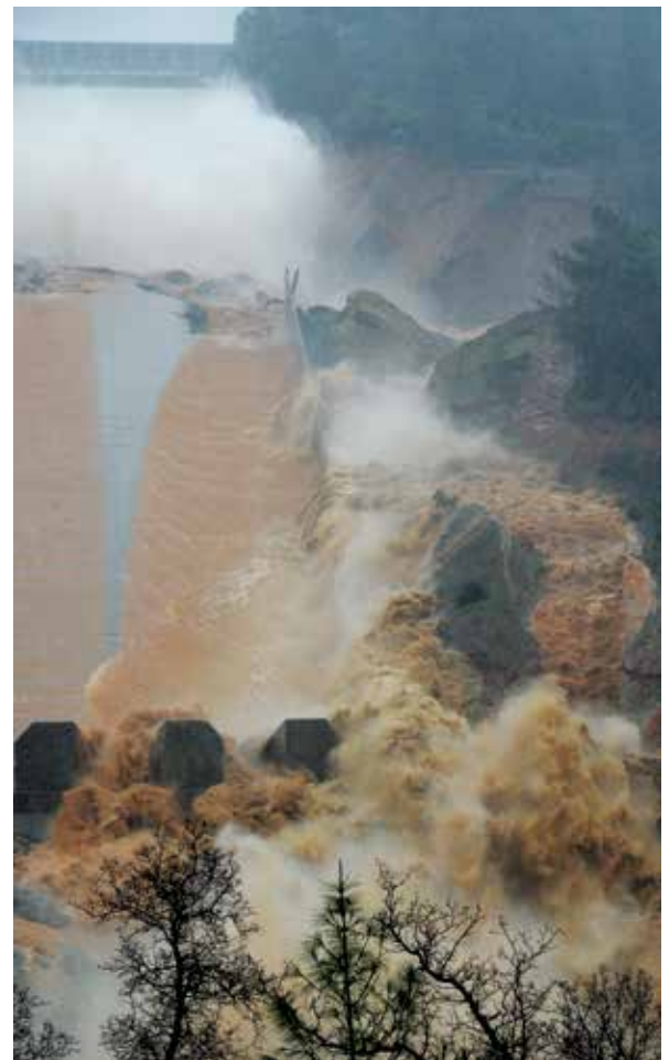
Damaged Oroville Main Spillway. Mud and debris tumble down the newly eroded channel alongside the Oroville main spillway on Feb. 8, 2017. Source: Bill Husa, Chico Enterprise-Record.
