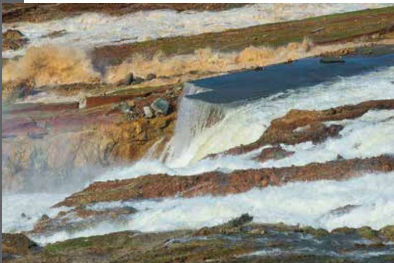
Emergency Spillway Flows and Erosion. Water flows over the Emergency Spillway for the first time on Feb. 12, 2017, eroding gullies and destroying a roadway. Source: Kelly M. Grow, DWR.
