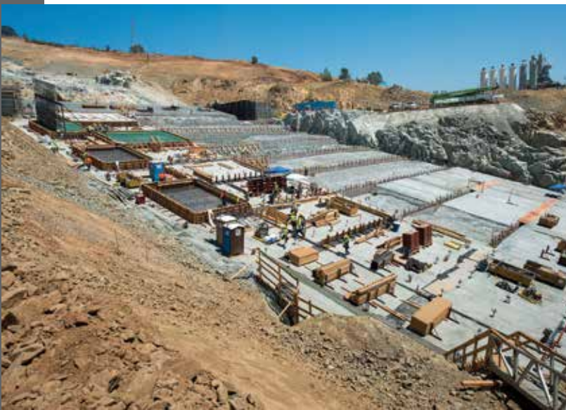
Oroville Dam Main Spillway Repair. Image date: August 9, 2017. Source: Florence Low, DWR.
