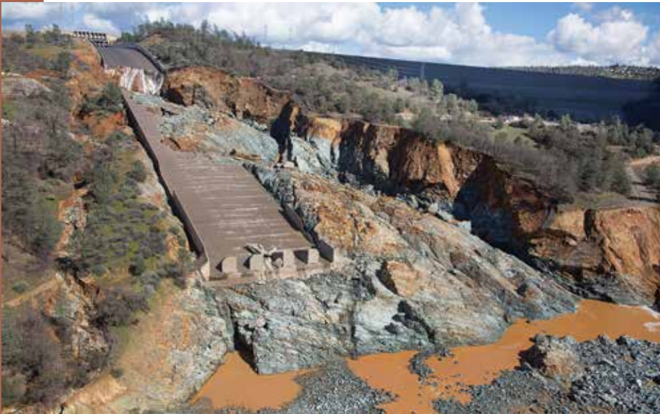
Oroville Dam Spillway, Feb. 27, 2017. The Oroville dam main spillway after spill flow releases ceased for repair inspections. Oroville Dam is in the shadow on the upper right. Source: Dale Kolke, CA Dept. of Water Resources (hereby DWR).
